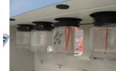
Bottle adaptors installed on the Illumina Analyzer
